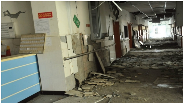
Damage and disruption
